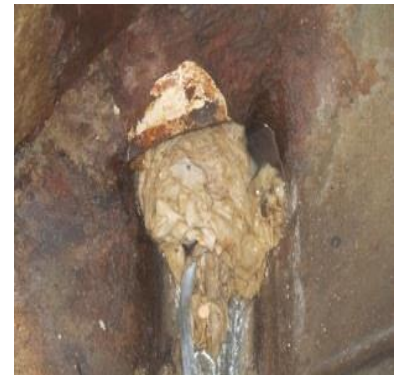
Accumulation of rags in the pipe.
